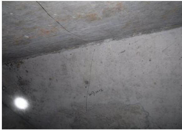
(a) 腹板斜裂缝
