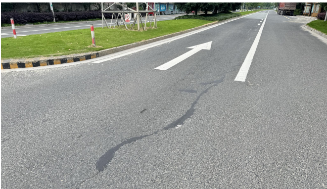
车辙、纵向裂缝
