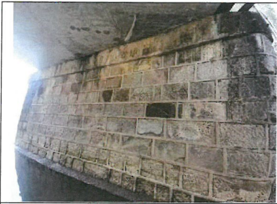
1#墩帽小桩号面雨水侵蚀
